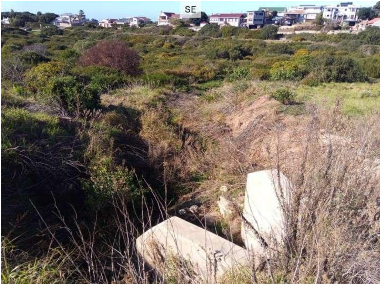
Figure 10. Example of the receiving environment showing storm water outlet with resulting erosion gully, vegetation cover and topography.
